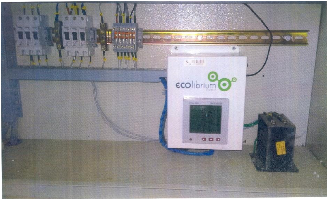
Smartsense energy meter integrated with main Incomer for meaurng energy consumption
