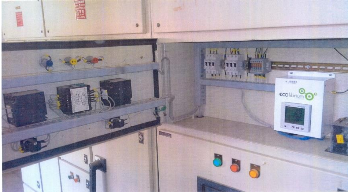
Smartsense energy meter installed at SIIB
